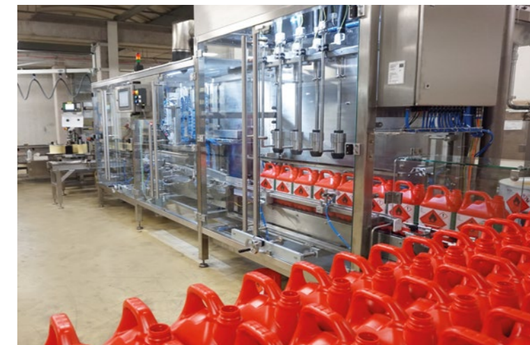
New filling system in the Oest hazardous goods workshop.
